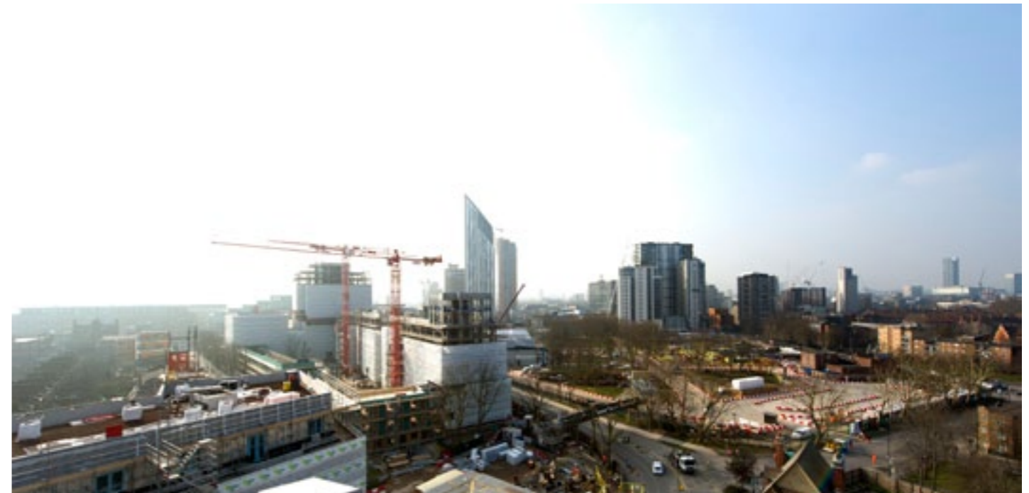
Elephant Park is progressing well with construction on South Gardens and West Grove now underway
